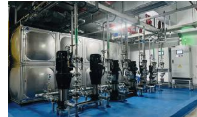
Boiler condensate water recovery project
